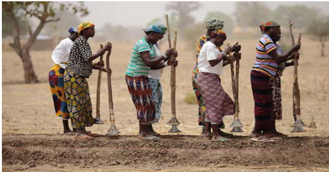
Women in Burkina Faso participate in a 'cash for work' project receive money for building embankments around fields to better irrigate crops during future dry seasons. Photo: Raphael de Bengy
